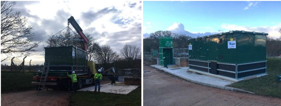
Figure 69 - Left: Dosing kiosk being lifted into position onto concrete plinth, Right: Dosing kiosk in location with nearby emergency shower
