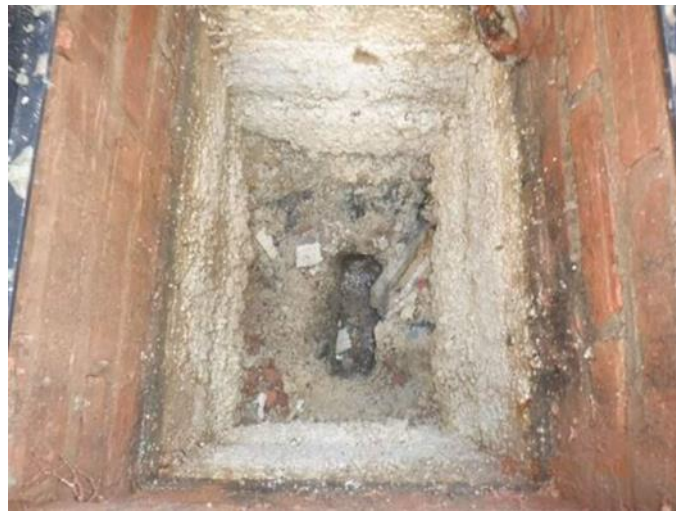
Figure 25 - Manhole downstream of food service establishments (FSEs), with elevated FOG levels
