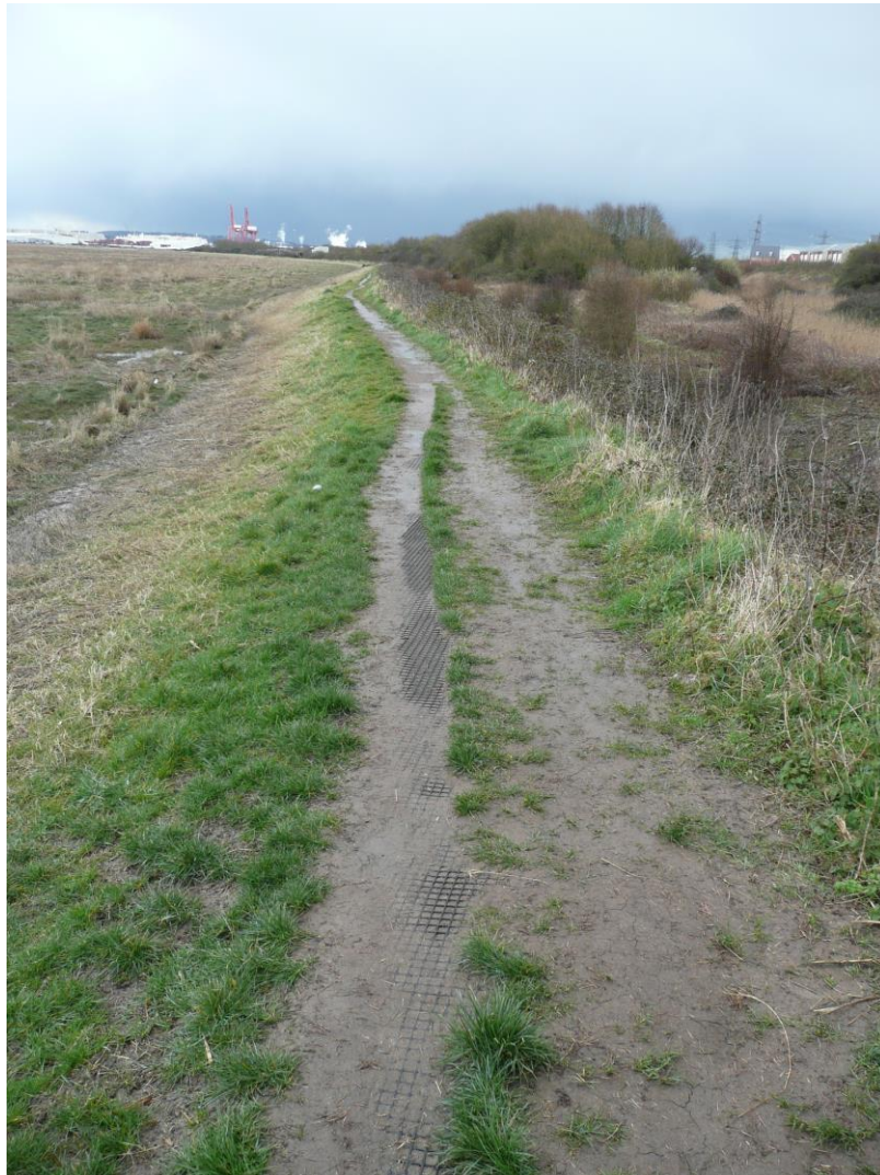
Figure 4. Exposed Geogrid on crest of wall
