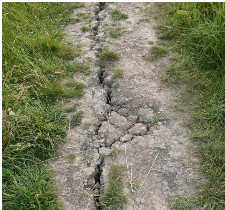
Figure 1. Longitudinal Cracking on crest of wall in dry conditions
