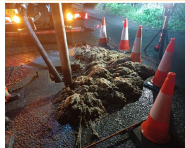
Wet wipes removed from a sewer in Highbridge, Somerset in March 2023.
