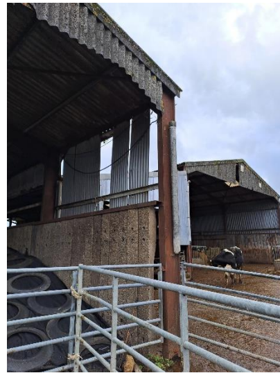
Broken guttering and downpipes that can be replaced. Photo credit: Tom Hicks
