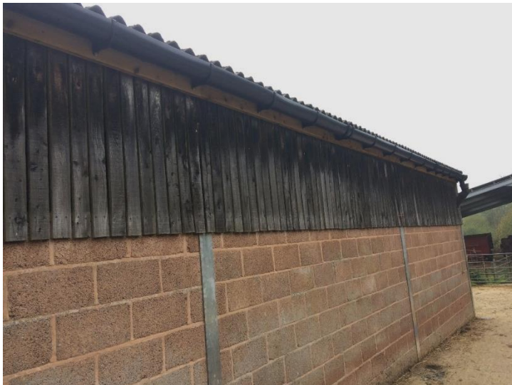
New guttering and downpipe on an existing cattle shed where the previous guttering was broken. Photo courtesy of Brinkworth Brook catchment advisor.
